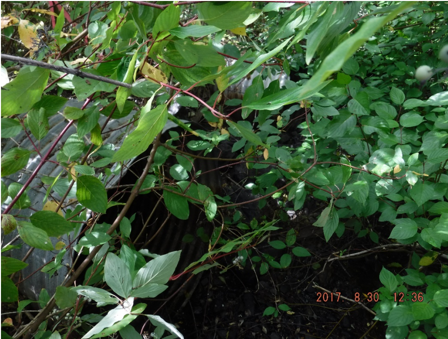
Photo II-47 Inlets of Ed Creek culverts under Pinchi Lake Road. Vegetation is not currently blocking the inlet but could become mobilized during flood conditions.
