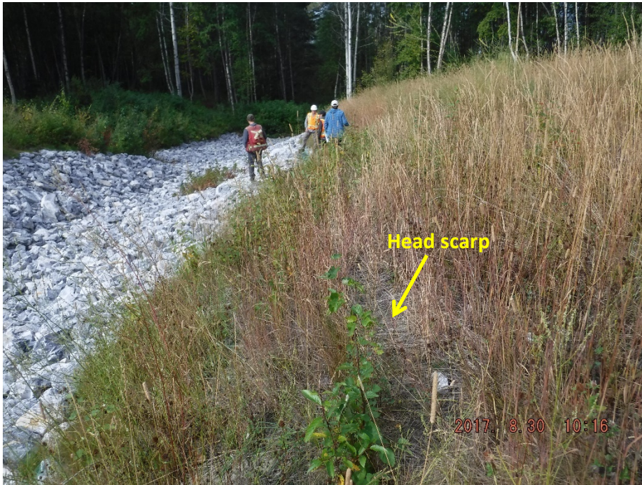
Photo II-23 Closure Spillway – head scarp of slump above right bank
