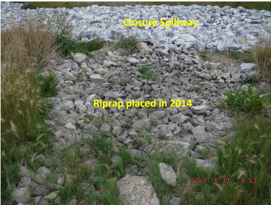
Photo II-20 Downstream end of surface runoff channel where it discharges to the Closure Spillway, showing riprap which was placed in 2014.
