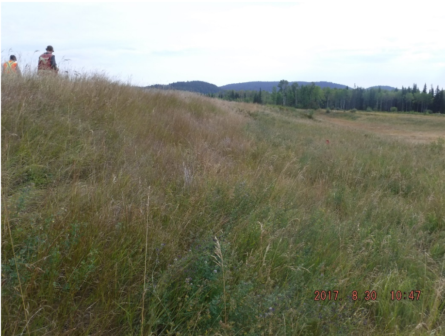
Photo II-6 Tailings Dam – South Leg, looking east along toe towards Borrow Area A.
