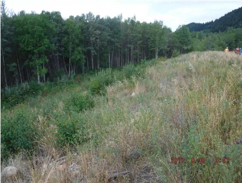
Photo II-13 Tailings Dam – Southwest Leg, looking northwest along dam slope towards corner with West Leg.
