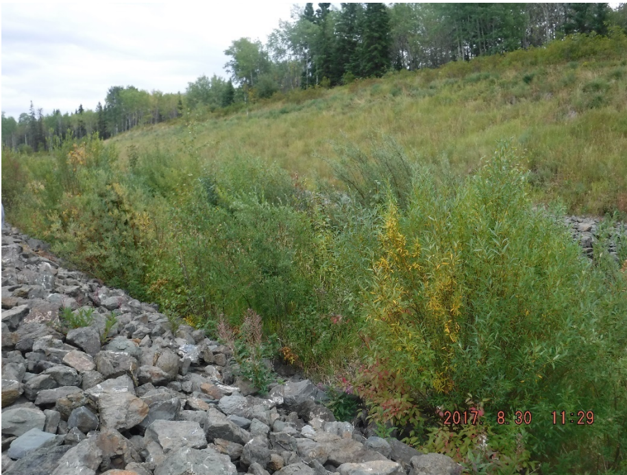
Photo II-39 Ed Creek Diversion Channel, looking upstream from near third bend. Channel base is covered with thick vegetation.
