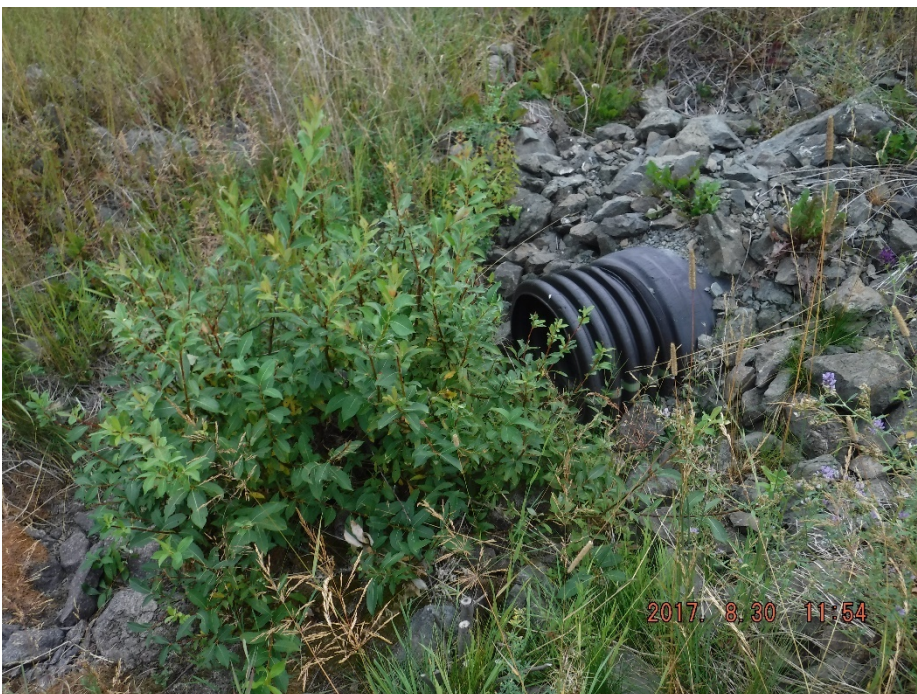
Photo II-46 Inlet of 460 mm culvert on north bank of Ed Creek Diversion Channel. There is vegetation upstream of the inlet that could block the channel during flood conditions.
