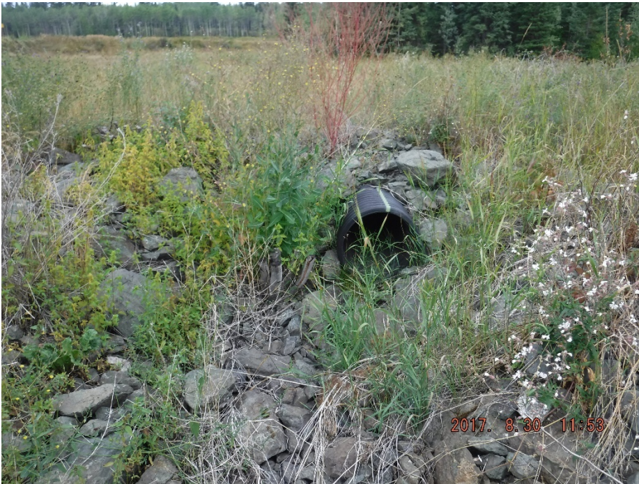
Photo II-45 Outlet of 460 mm culvert on north bank of Ed Creek Diversion Channel.
