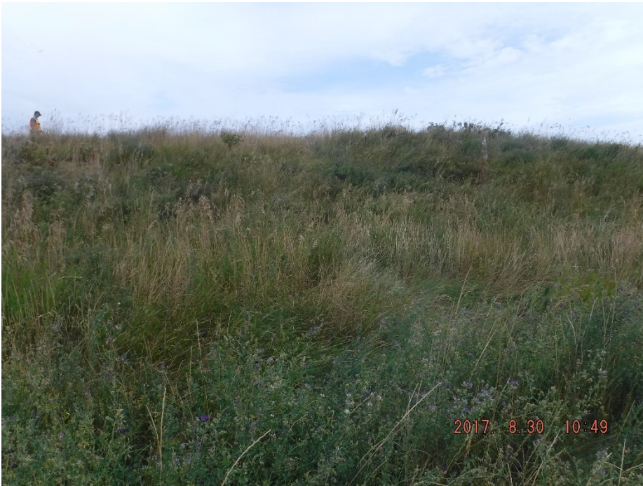
Photo II-7 Tailings Dam – South Leg, looking up the slope from the toe area.
