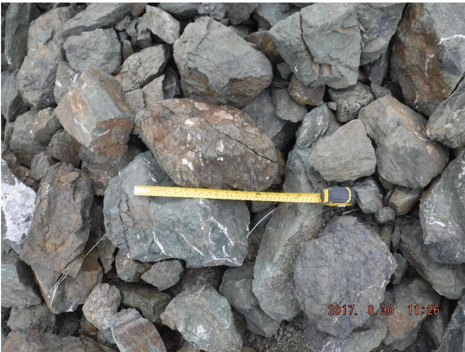
Photo II-38 Ed Creek Diversion Channel – Riprap on right bank, showing weathering and breakage
