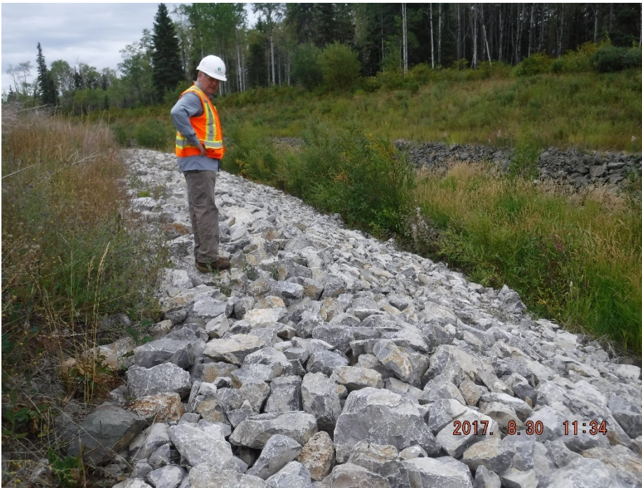
Photo II-41 Ed Creek Diversion Channel – area on right bank where riprap was replaced in 2014. Riprap in this area is in good condition.
