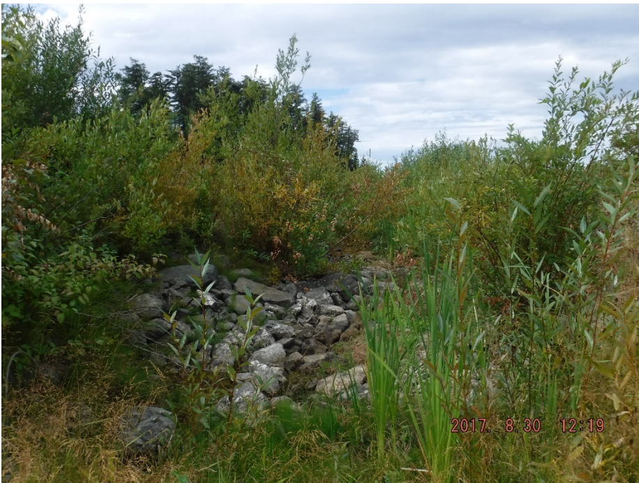
Photo II-30 Spillway Downstream Channel – Lower Reach, looking downstream from culvert beneath road to caretaker's house.
