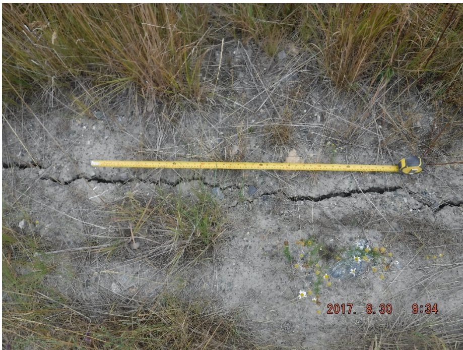
Photo II-10 Tailings Dam – Southwest Leg, crack on dam crest in tire track.
