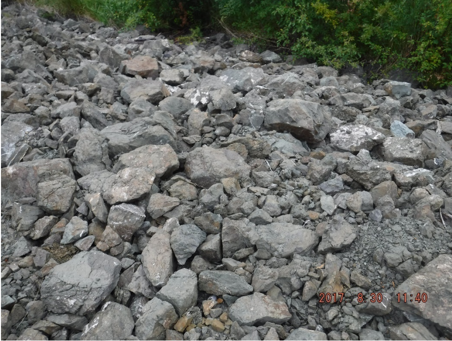
Photo II-43 Ed Creek Diversion Channel - Top of right bank where there is a depression in the riprap surface (location 9 in Figure 4.1), and riprap appears to be deteriorating more than other areas.
