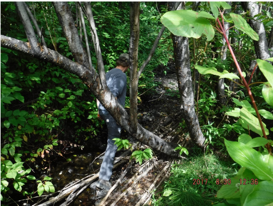
Photo II-48 Ed Creek culverts under Pinchi Lake Road, looking at channel upstream of culverts. There is debris in the channel.
