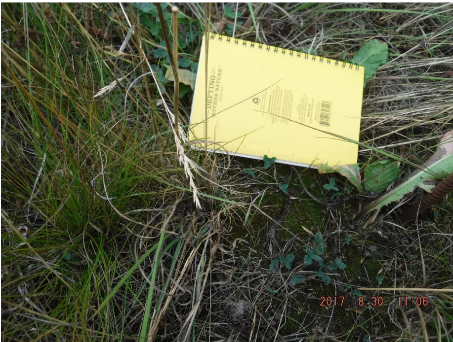
Photo II-32 Borrow Area A – tension crack on slope at monitoring rod location 403. Crack shows no sign of widening compared to previous inspections.
