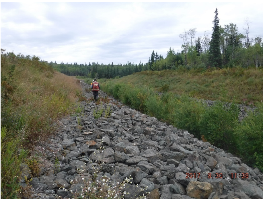
Photo II-42 Ed Creek Diversion Channel – looking upstream from near second bend towards depression in riprap surface (location 9 in Figure 4.1).
