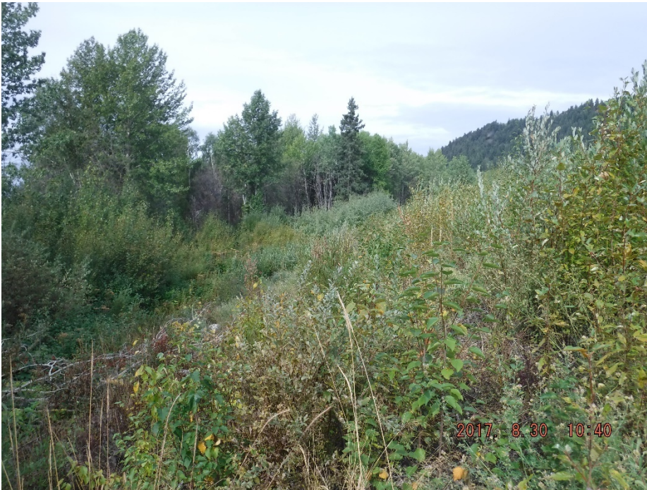
Photo II-14 Tailings Dam – Southwest Leg, looking northwest along dam slope from toe area.
