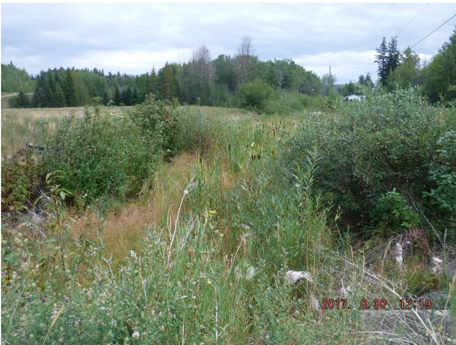
Photo II-28 Spillway Downstream Channel – Middle Reach, looking upstream from culvert beneath road to caretaker’s house.
